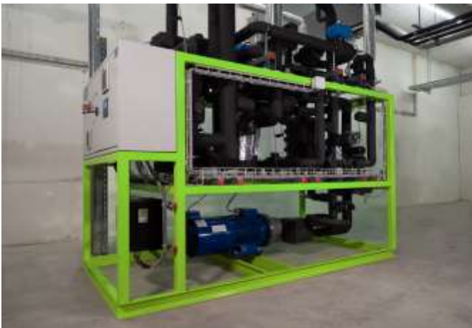
Figure 1: Energy-Transfer-System of Prodega Dietikon-Zurich, a world first unit in operation since autumn 2022.
